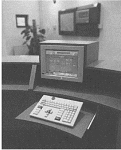
Figure 10.5 Fire detection central station (Courtesy of Gent & Co. Ltd)
